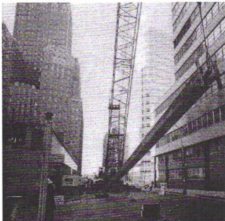
Caisson core on way into utility substation (left) tough to maneuver on narrow street.
